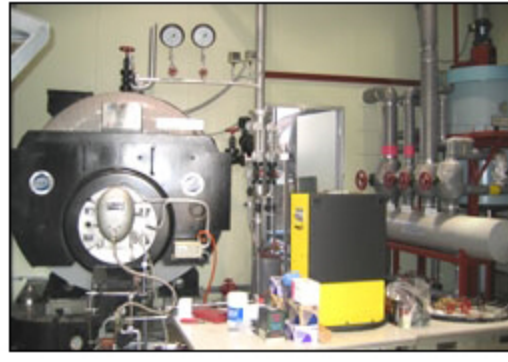
Boiler for testing reduction of particles in heavy oil(1.5ton)
