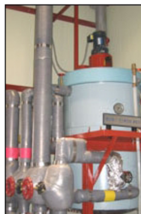
Mixing tank for mixing the fuel additive for heavy oil
