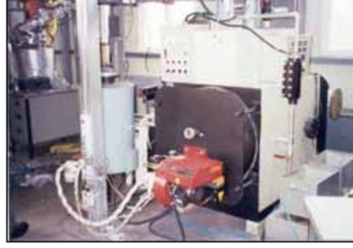
Boiler for testing fuel additive performance
